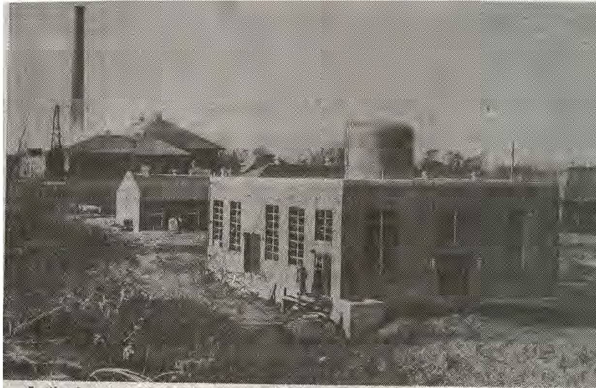
In the foreground, is the new pumping station which takes the water from the lake and into the filter system. The new pumps will make it possible to clean 25 filters at once instead of 10 as with the facilities in use for years. When the water in the lake is down the pumps go into operation.
